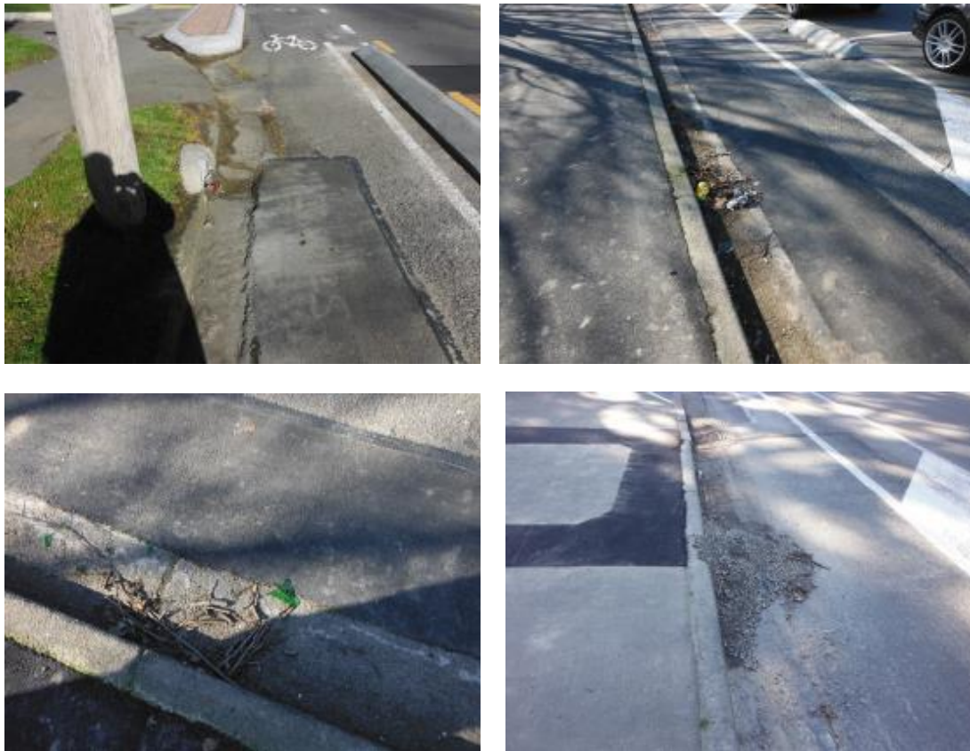
Figure 2-9: Note uneven surface and debris in cycle lane
