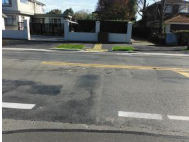
Figure 2-5: Example of Bitumen Flushing
