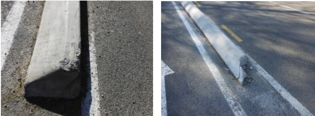
Figure 2-6 Note damaged kerbs and missing reflective studs
