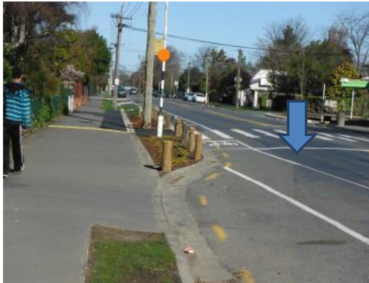
Figure 2-4: Note binder rich surface on approach to the crossing.
