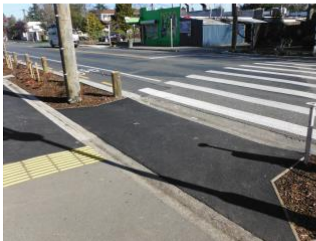
Figure 2-2 Zebra Crossing north of Rountree St. Note missing tactile paving
