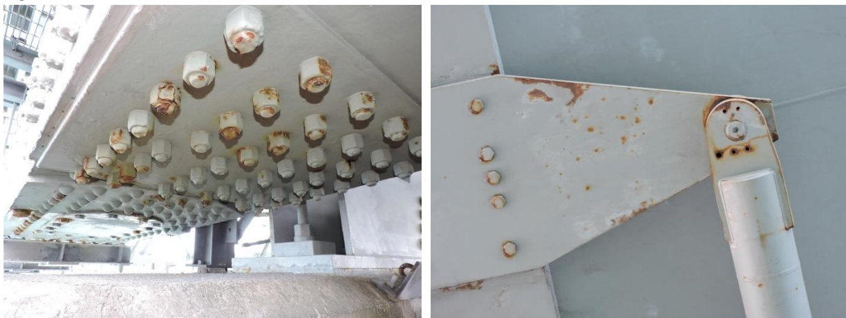
Figure 4-2: Example of substrate corrosion.
