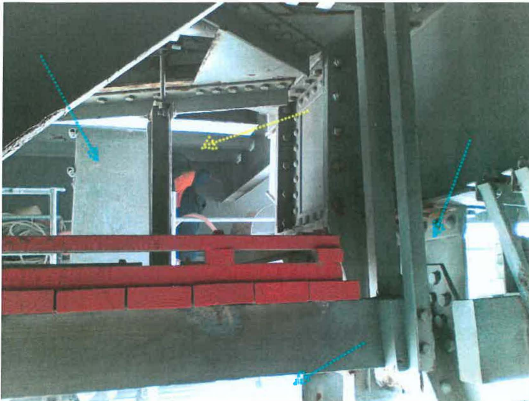
Photo 2 Gaps in bridge structure through which dust cloud penetrates
