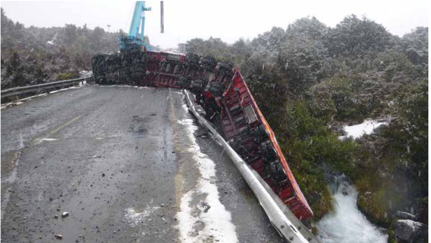
The Waihohonu Stream Bridge was damaged in a truck crash last winter
