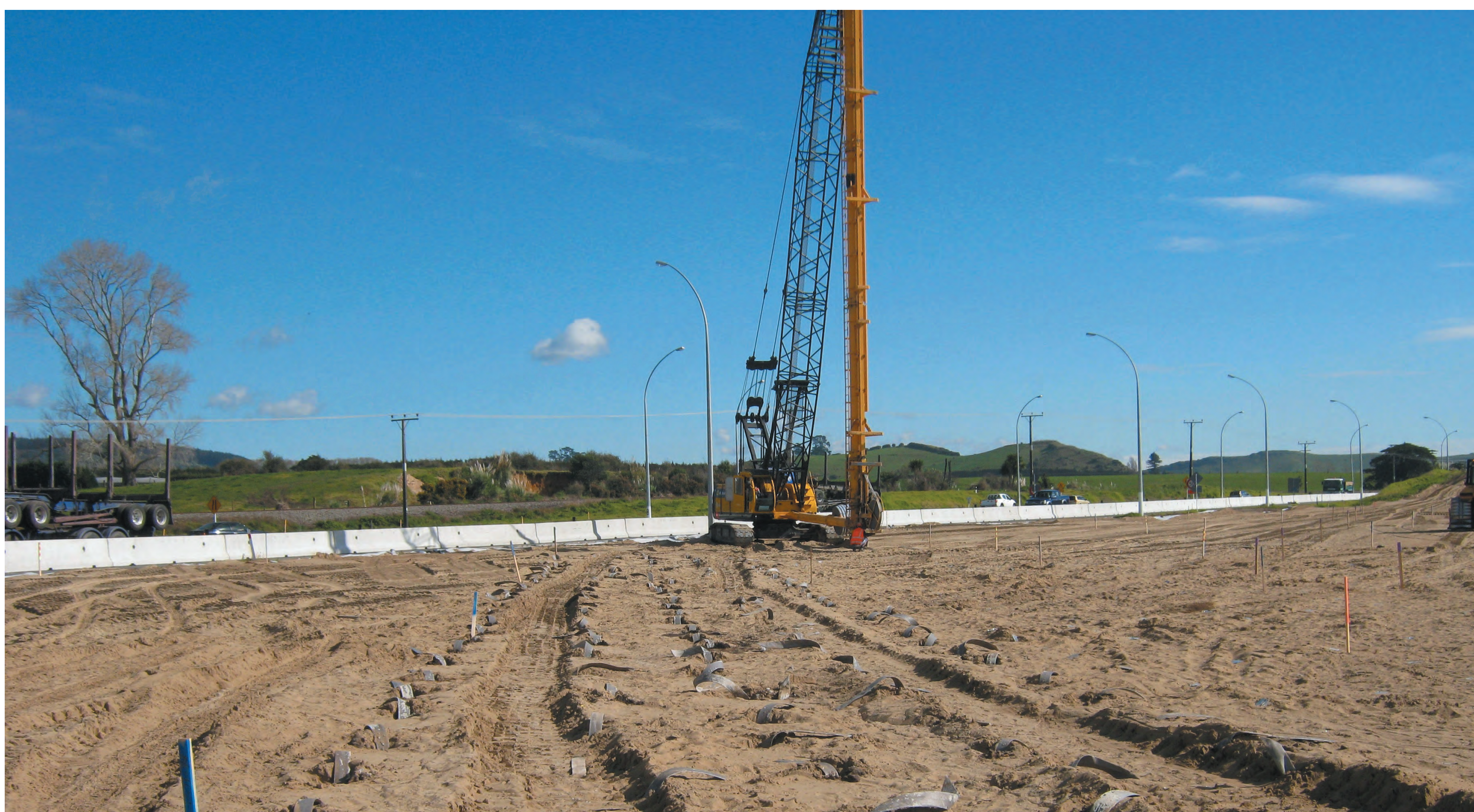
Wick drilling: A crane is used to insert the wicks up to 25 metres into the ground.
