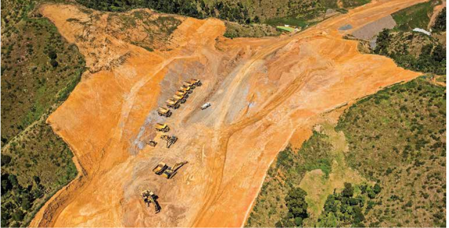
At the summit, deep into the cutting, greywacke rock is clearly visible.
