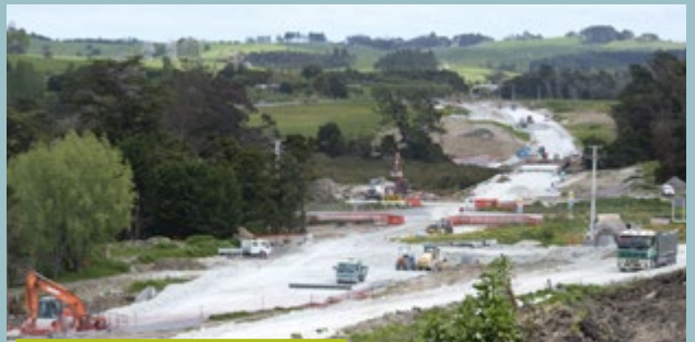
Earthworks either side of the state highway where the realignment crosses it near Anderson Bridge. There'll be a series of staged traffic switches from early 2019, including to allow works to continue where the realignment intersects with the existing state highway and to build the new intersection leading into Matakohe township
