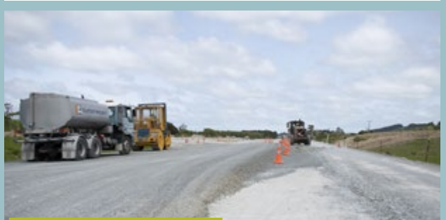
The pavement crew are building up the road using aggregate which is compacted in layers on top of the limestone subgrade, works at western end of realignment pictured
