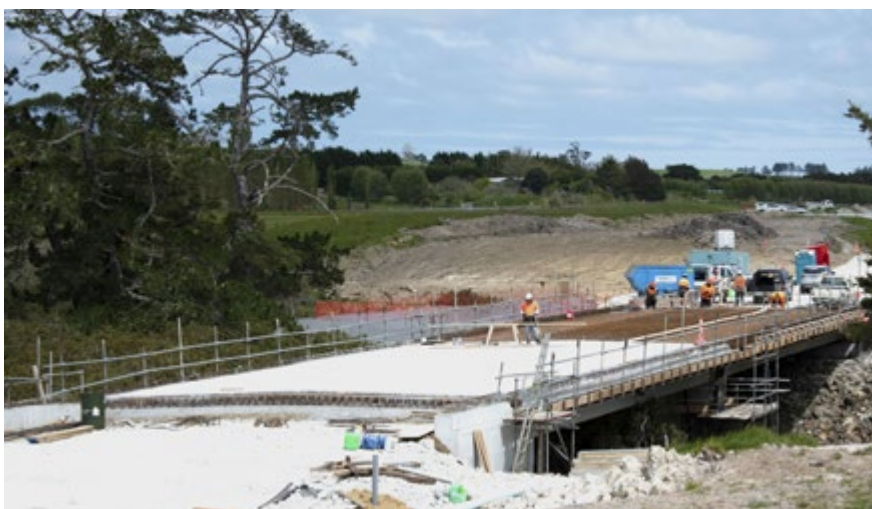
Bridge No.1's full deck has now been poured and the bridge barriers are being installed, eastern side of the deck poured pictured
