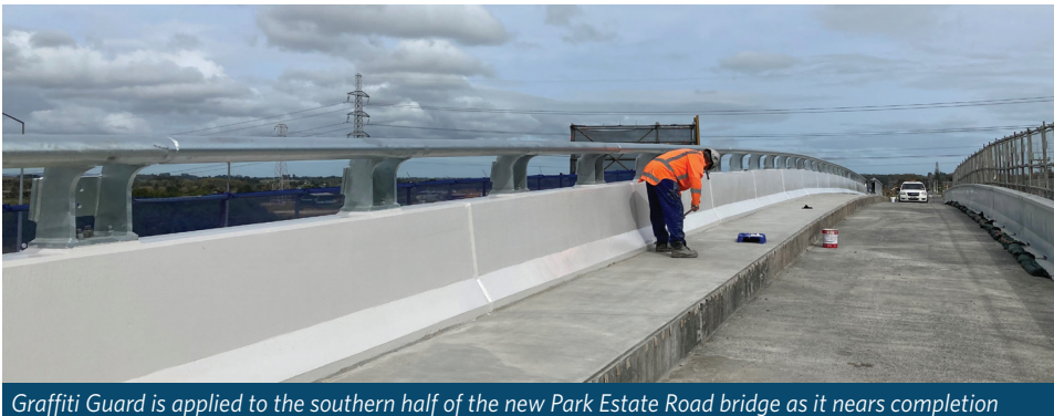
Graffiti Guard is applied to the southern half of the new Park Estate Road bridge as it nears completion
