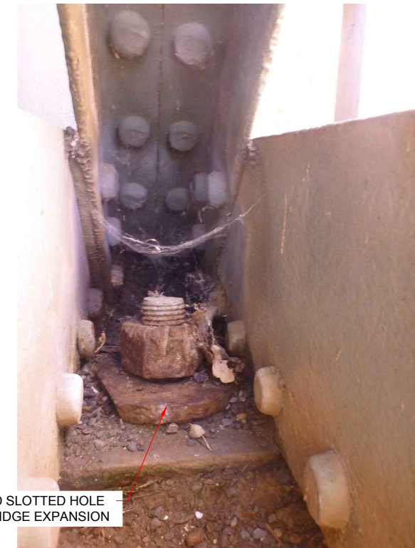
REMOVE NUT AND WASHER FROM HOLD DOWN BOLTS AT ABUTMENT A AND CUT A LARGER SLOTTED HOLE IN THE BASE PLATE TO ALLOW THE TRUSS TO SLIDE BACK FURTHER TOWARDS THE ABUTMENT BACK WALL, EXTEND HOLE BY APPROX 50mm, EXTENT TO BE CONFIRMED ON SITE BY ENGINEER. ONCE NUT AND WASHER HAVE BEEN REMOVED. REINSTATE WASHER AND NUT.
