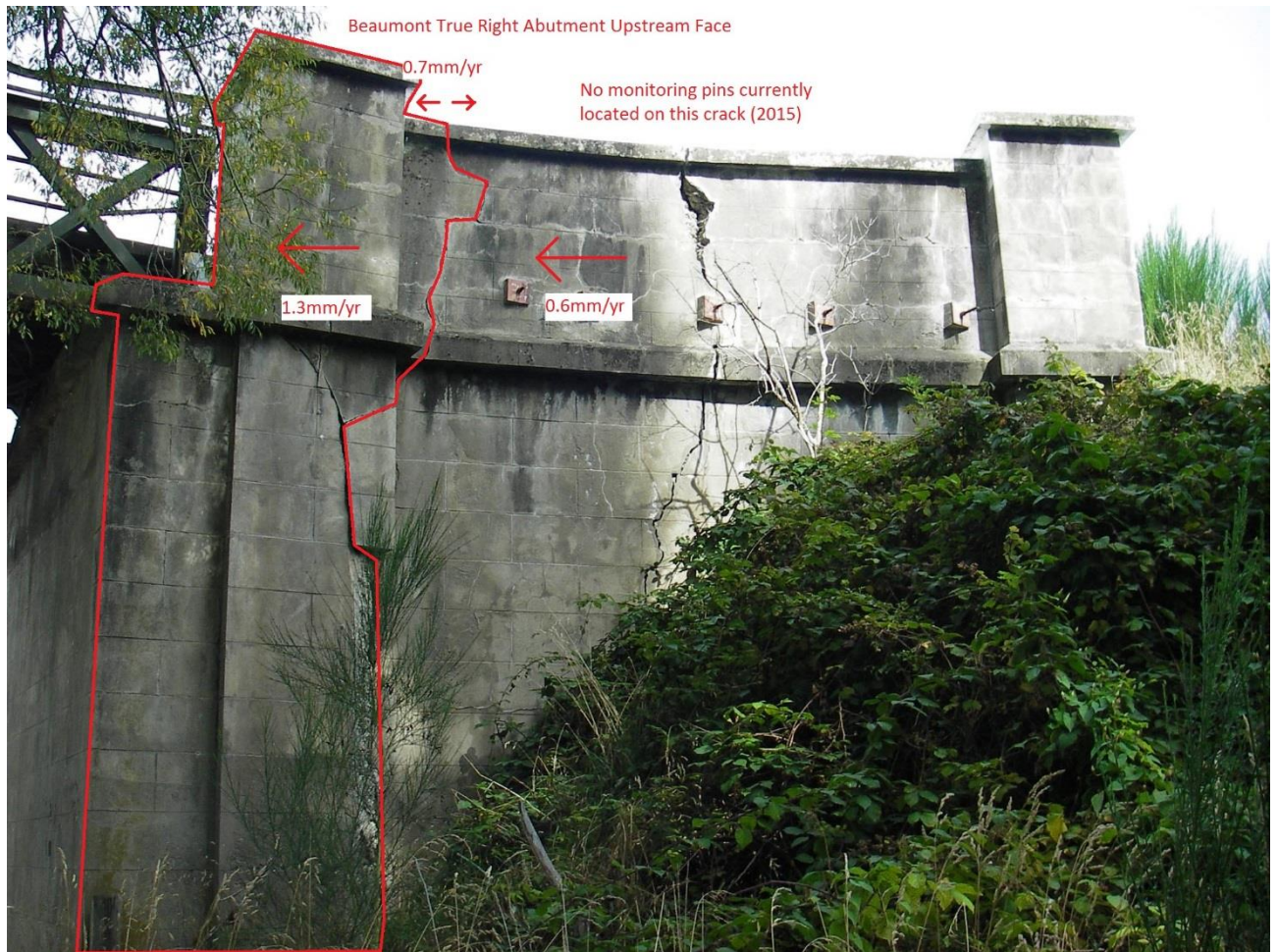
Figure 3 – Cracking and creep movements observed (December 2015, Opus)
