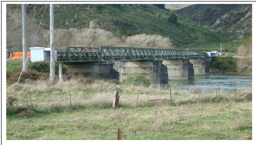
SH8 Beaumont Bridge (Pre-scaffold) Photo looking West (Alexandra end) to East (towards Milton SH 1)
