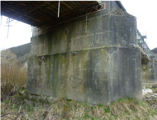
Figure 31: Concrete pier. Staining, microbiological growth, cracking, and graffiti are visible.
