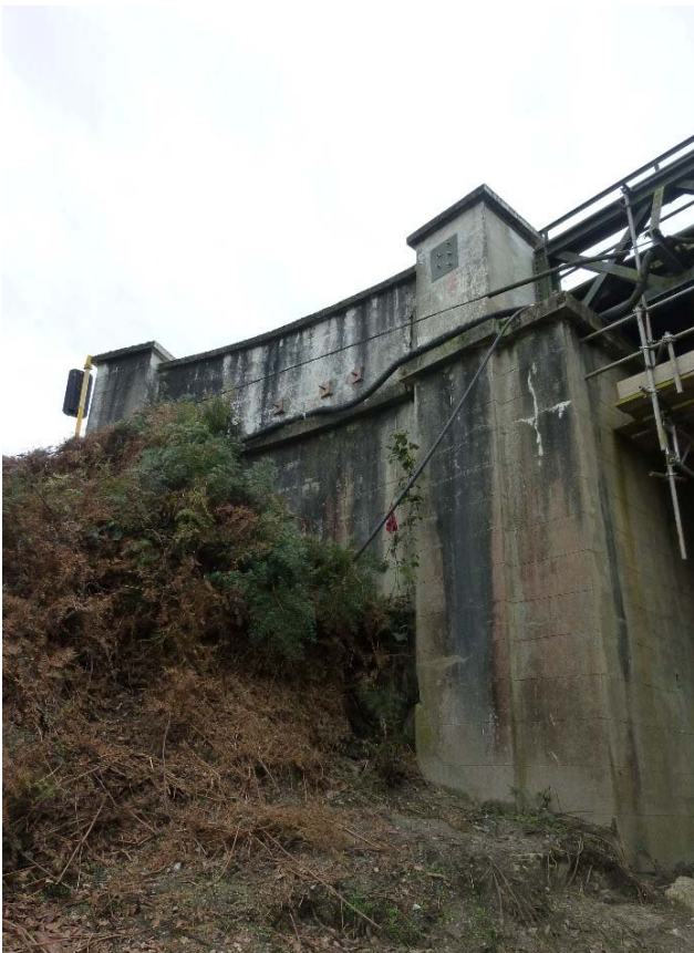
Figure 29: South elevation of west abutment. Staining, microbiological growth and cracking are visible. Note also the strengthening works that have been carried out.
