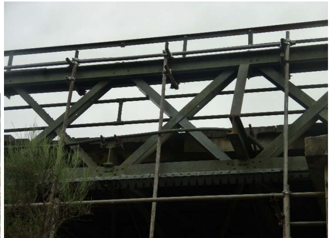
Figure 32: Lattice girder behind scaffold. Transom ends are visible, intersecting with bottom chord.
