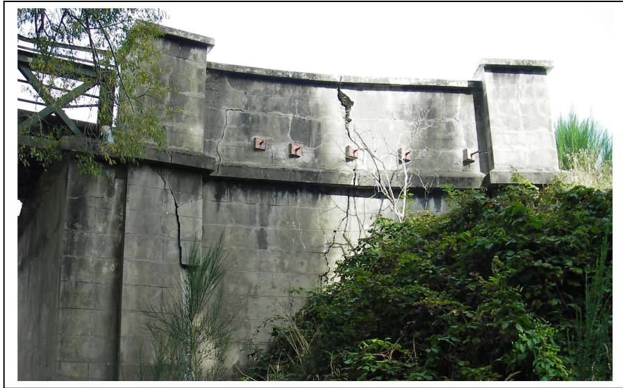
Western Abutment Settlement
