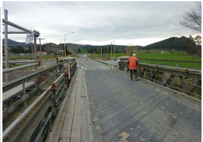
Figure 34: Bridge deck looking west. The poor condition of the deck surface is evident.
