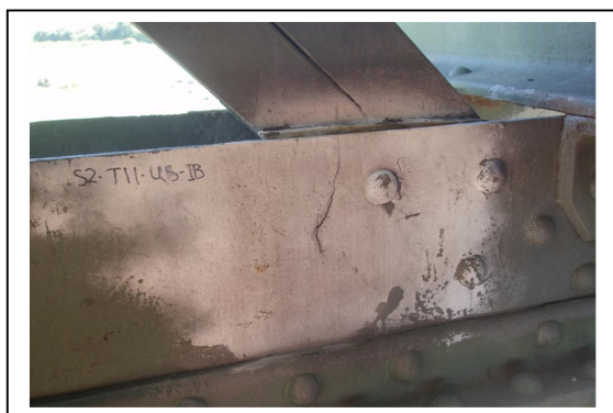
Surface Star Cracking
