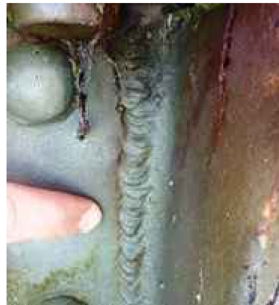
CRACK AT TOP OF WELD
