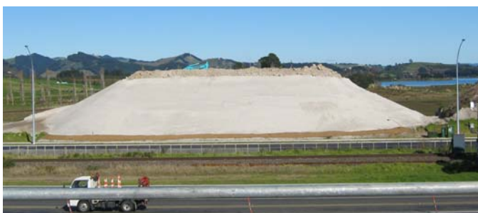
Mangatawa interchange (Truman Lane side) embankment fill material now completed with pre-load rubble on top.
