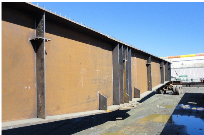
Below: One of the Kaituna River bridge steel girders at the Eastbridge yard, in Napier.
