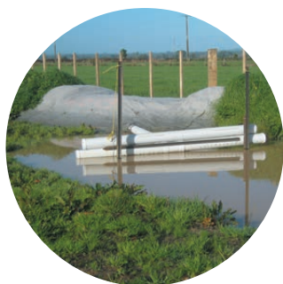
Decanting earth bund ensures only treated water enters the surrounding drainage system
