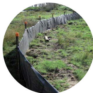
Silt fences are used to limit silt from entering the surrounding drainage system
