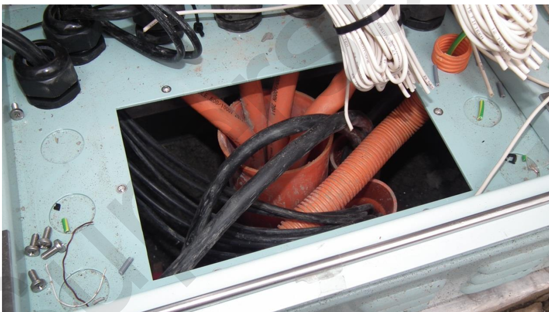
Figure L02 -Bottom of controller cabinet with gland plate access panel removed
