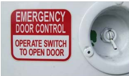
Operating instructions (outside) on a power operated door used as an emergency exit.
