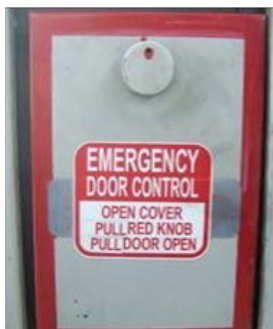
Door operating instructions (inside) by the door.
