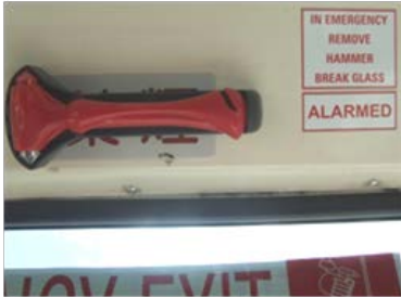
Glass breaking device (hammer) securely fitted next to the breakable glass.
