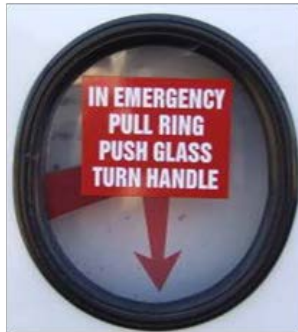
Pull ring gone missing.
