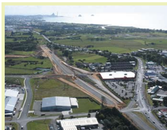
Looking towards New Plymouth, work continues on the $20.2m Bell Block bypass.
