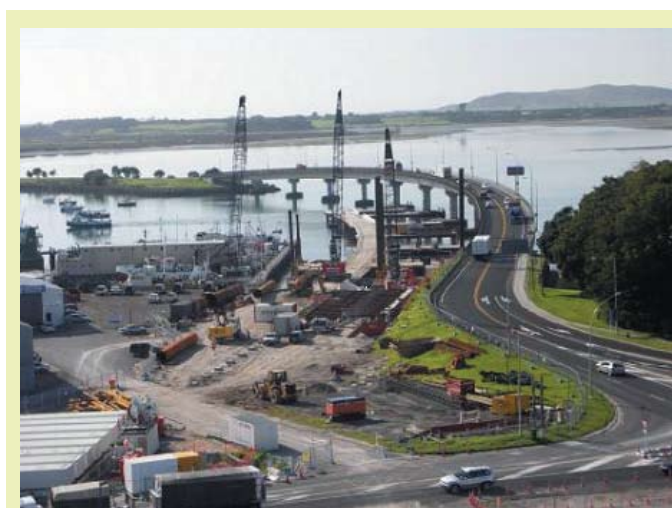
Work is progressing on the construction of the new bridge as part of the Tauranga Harbour Link project.
