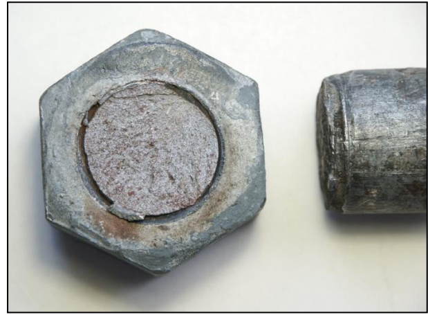
Figure 45. Failure at bar head on bridge.
