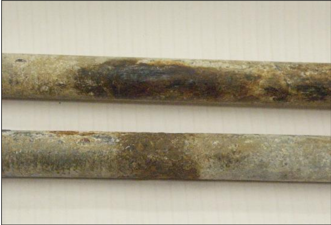
Figure B4. Corrosion on Ahuriri River Bridge linkage bolt.
