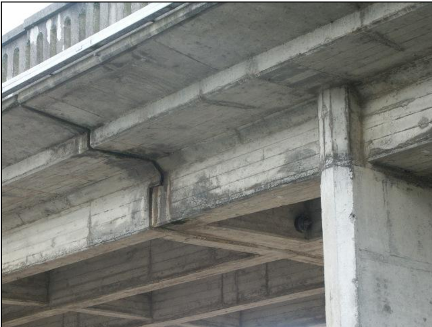
Figure 66. Otaki River Bridge. Details of in-span hinge are shown in the bottom photo.
