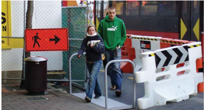
Photo 18.6 – Footpath diverted onto protected roadway with temporary kerb crossing and rail (Photo: Tim Hughes)
