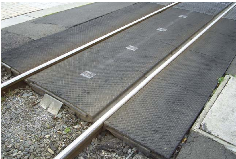
Photo 15.27 – Rubber crossing surface, Tauranga (Photo: Greg Hackett)
