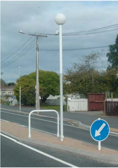
Photo 15.6 – Pedestrian island lighting column and globe, Hamilton (Photo: Shaun Peterson)
