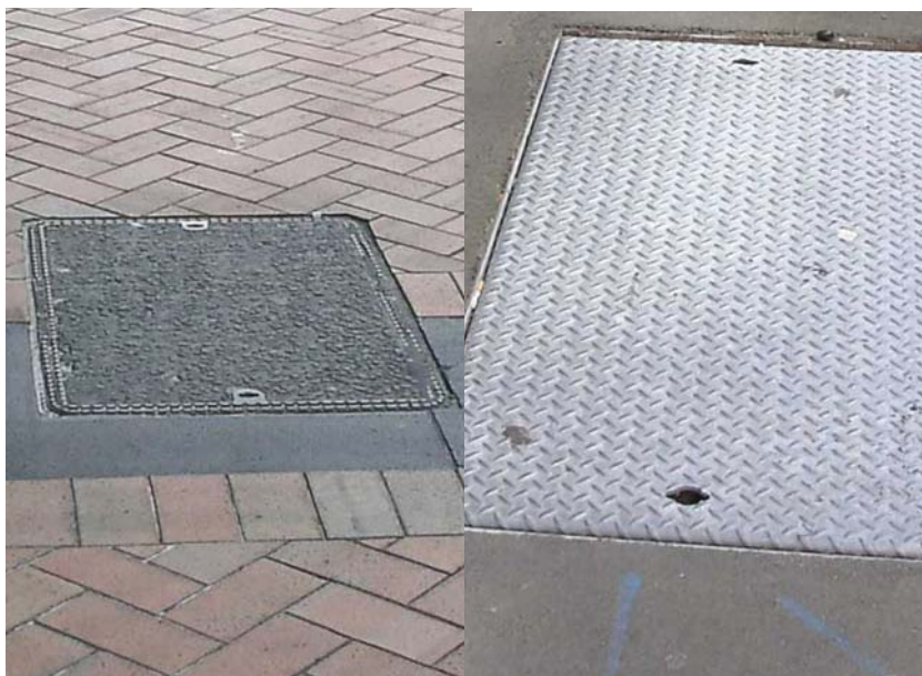
Photos 14.8 & 14.9 – Covers in through route, Wellington (Photo: Shane Turner)
