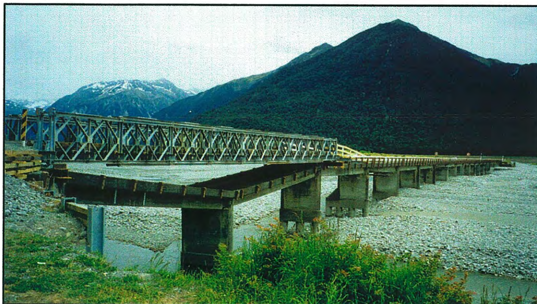
Figure 3.2 Failed spans at the Bealey (eastern) end of the bridge.
