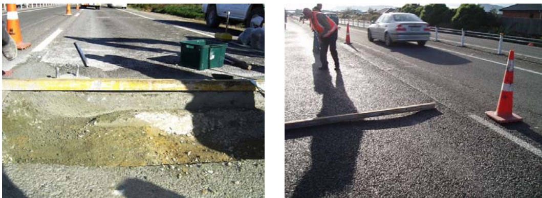
Figure 3.2 Trenched profile (left) and rutting under straight edge (right)
