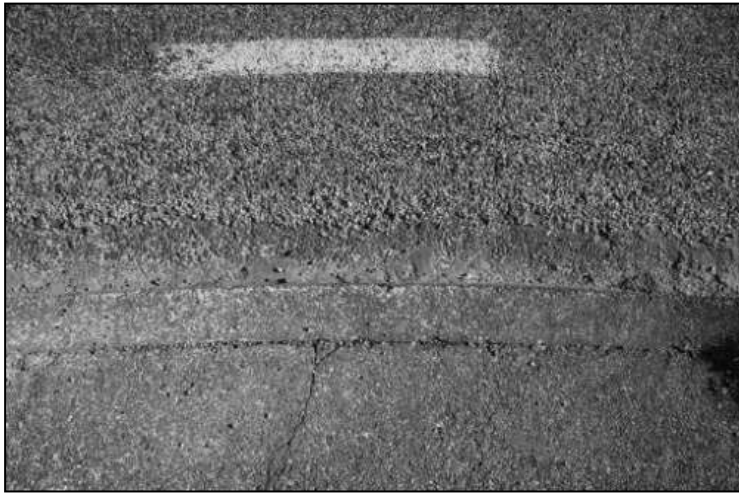
Figure B2 Close-up view of accident site 1
