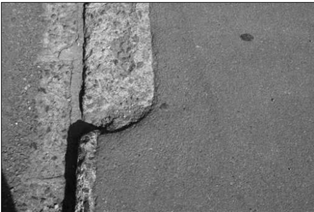
Figure B8 Close-up view of accident site 4
