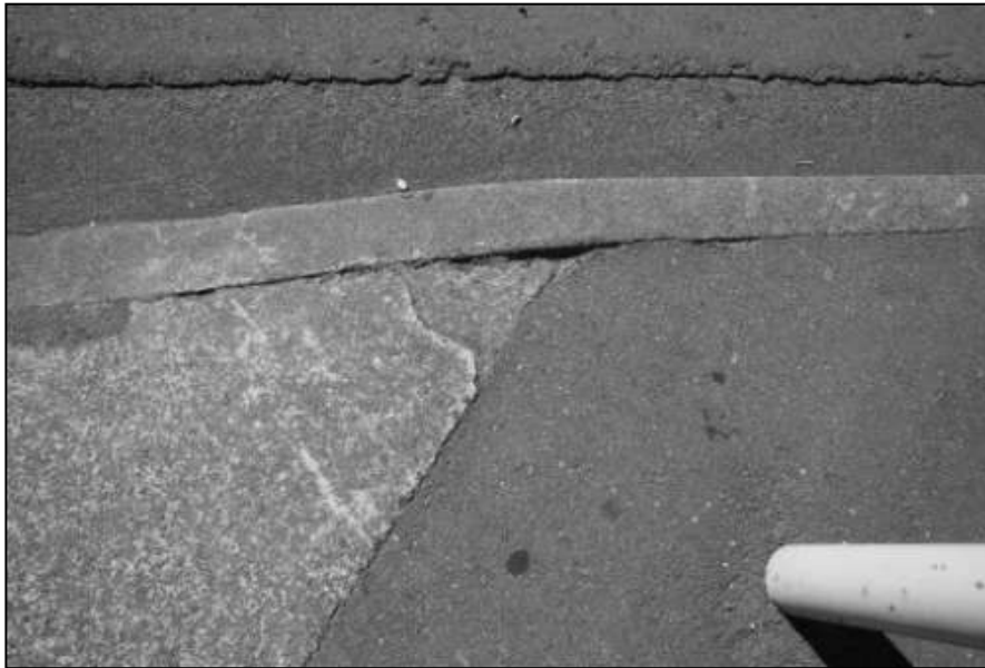
Figure B12 Close-up view of accident site 6
