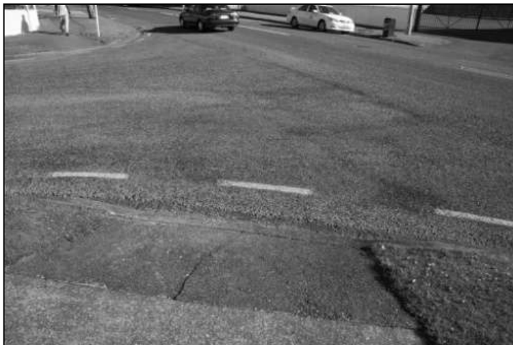
Figure B1 Long-shot view of accident site 1
