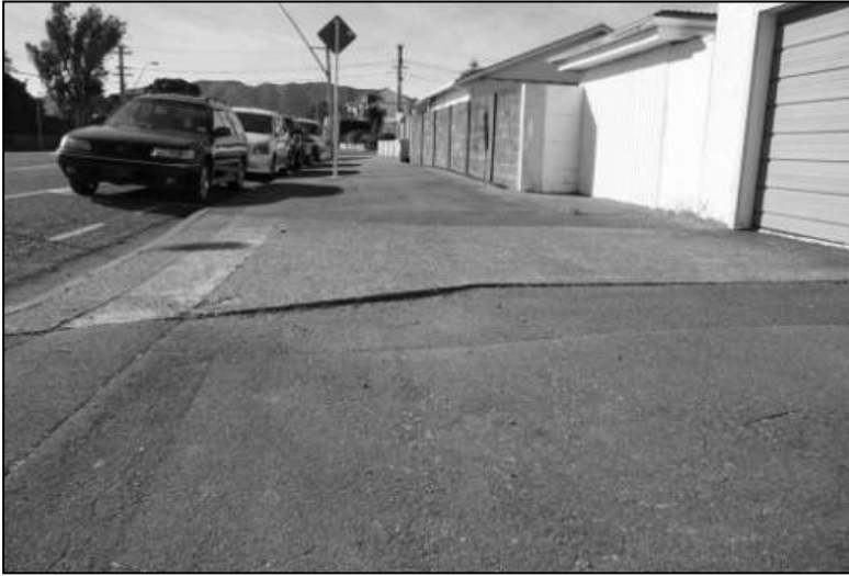
Figure B3 Long-shot view of accident site 2
