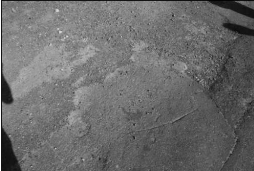
Figure B6 Close-up view of accident site 3
