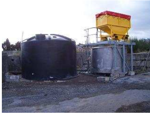
Figure 1 – CMA Mixing and Storage Facility
